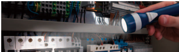
Erroneous circuit-breaker activation
